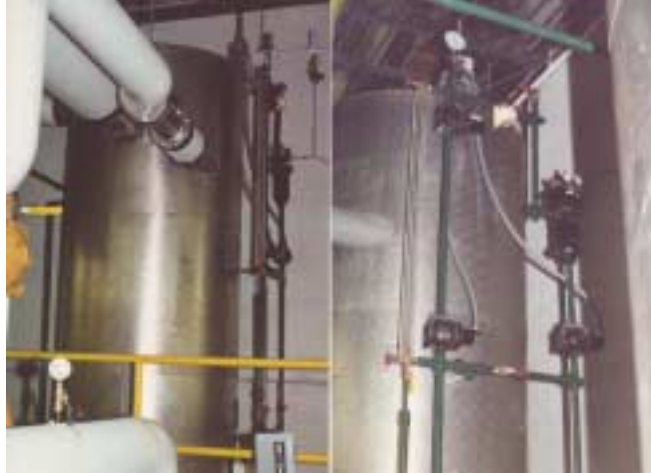
Figure 7: Heat Recovery Equipment
