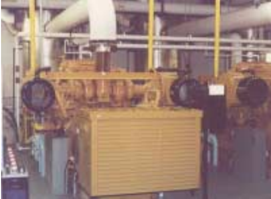
Figure 2: Caterpillar Engine Generator Set
