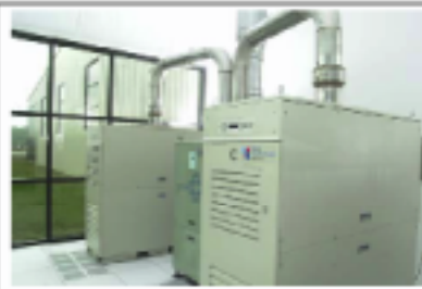
The Microturbines and Heat Exchanger
