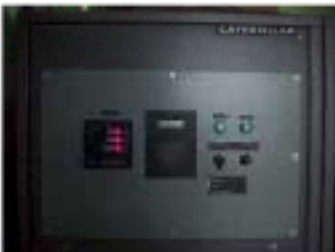
Engine Control Panel
