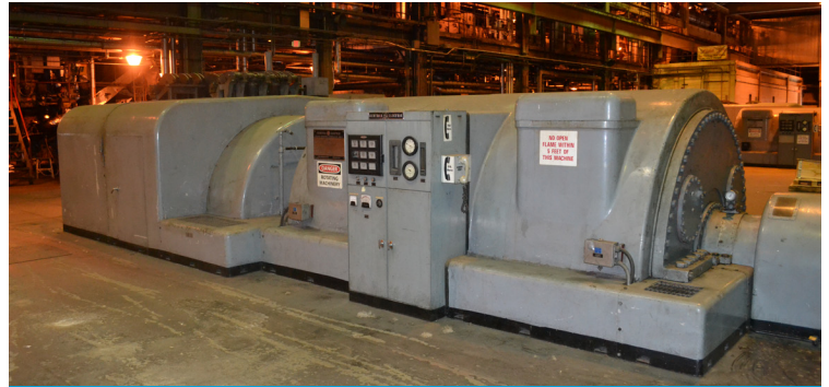
Steam turbine CHP installation at an industrial facility in New York. Photo courtesy of Recycled Energy Development
